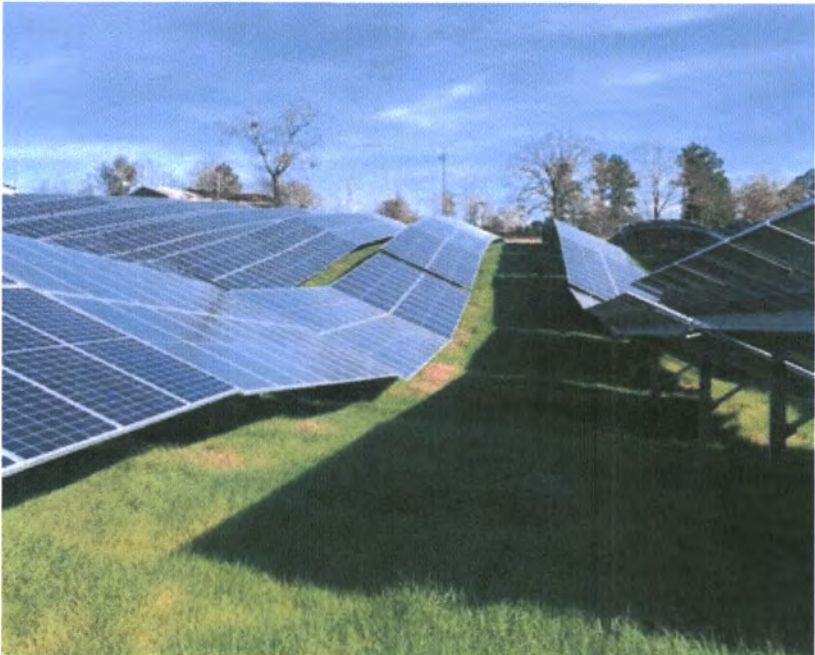
SolAmerica Fixed Tilt Project (installed in 2018)
