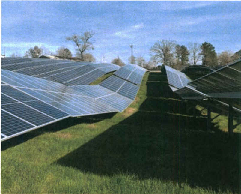
SolAmerica Fixed Tilt Project (installed in 2018)
