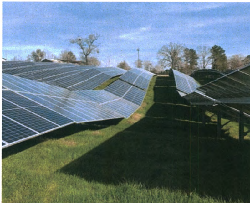
SolAmerica Fixed Tilt Project (installed in 2018)
